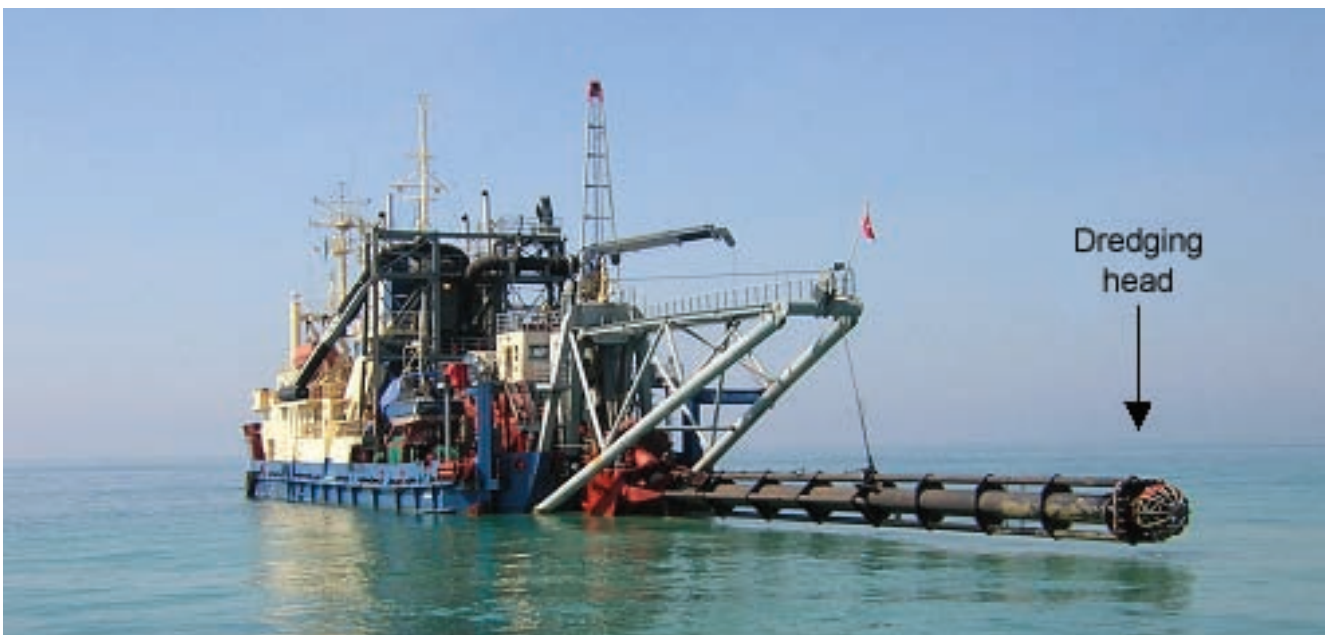
Figure 1.4 - Anchor dredging with superficial pipe; the dredging head is visible on top of the pipe.
