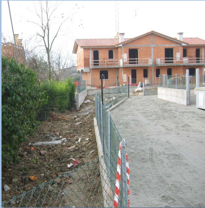
Ditch cover = loss of drainage capacity
