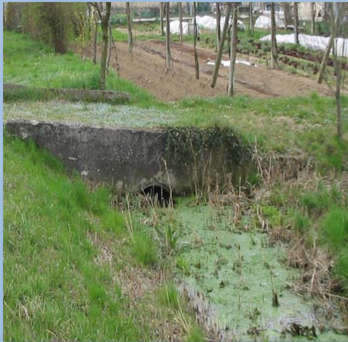
With pipes = section reduction – drainage problems
