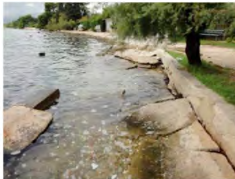
Broken coastal constructions
