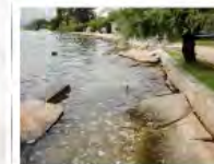
Broken coastal constructions
