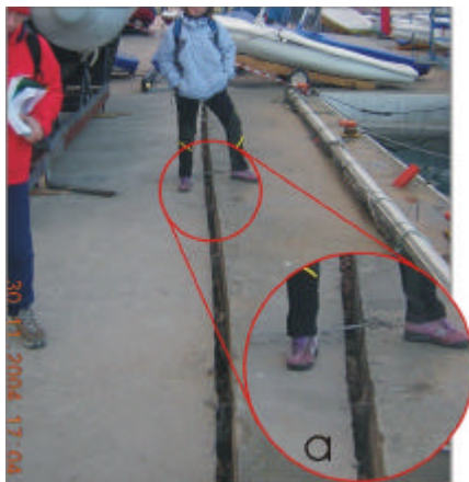
Figure 2: Fissure parallel to the waterfront, affecting the concrete in the Salò harbor area. This feature is an evidence of liquefaction and localized lateral spreading.
