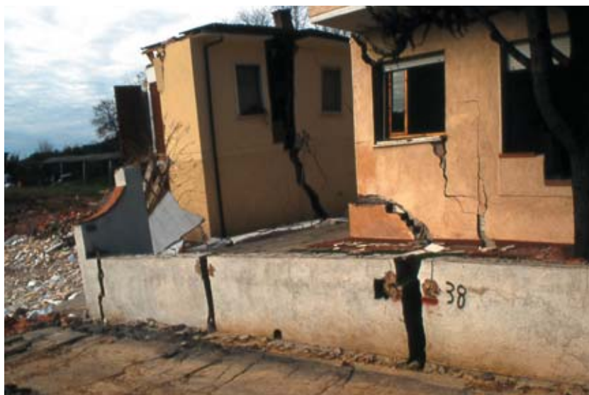
Fig. 2 - Edifici semidistrutti presso la voragine. Half-destroyed buildings close to the sinkhole.
