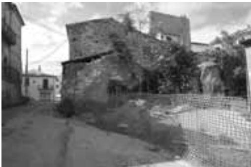
Figure 2.6 - Damage along a reactivated scarplet.
