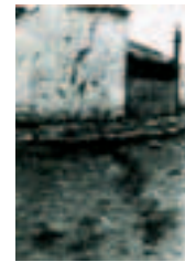
Figure 2.2 Earthquake induced ground fracture, cutting a house
