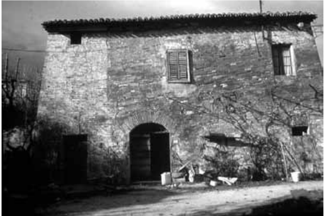
Figure 5.11 - A 16 th century post-house, showing the cumulative effects of recurrent landslide movements on the Montagnolo slope.
