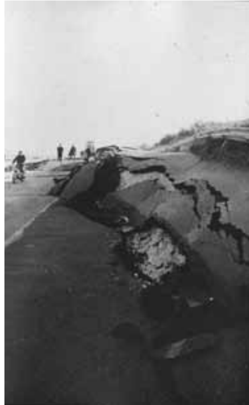
Figure 5.10 - Damage to the Adriatic railway at the landslide toe.
