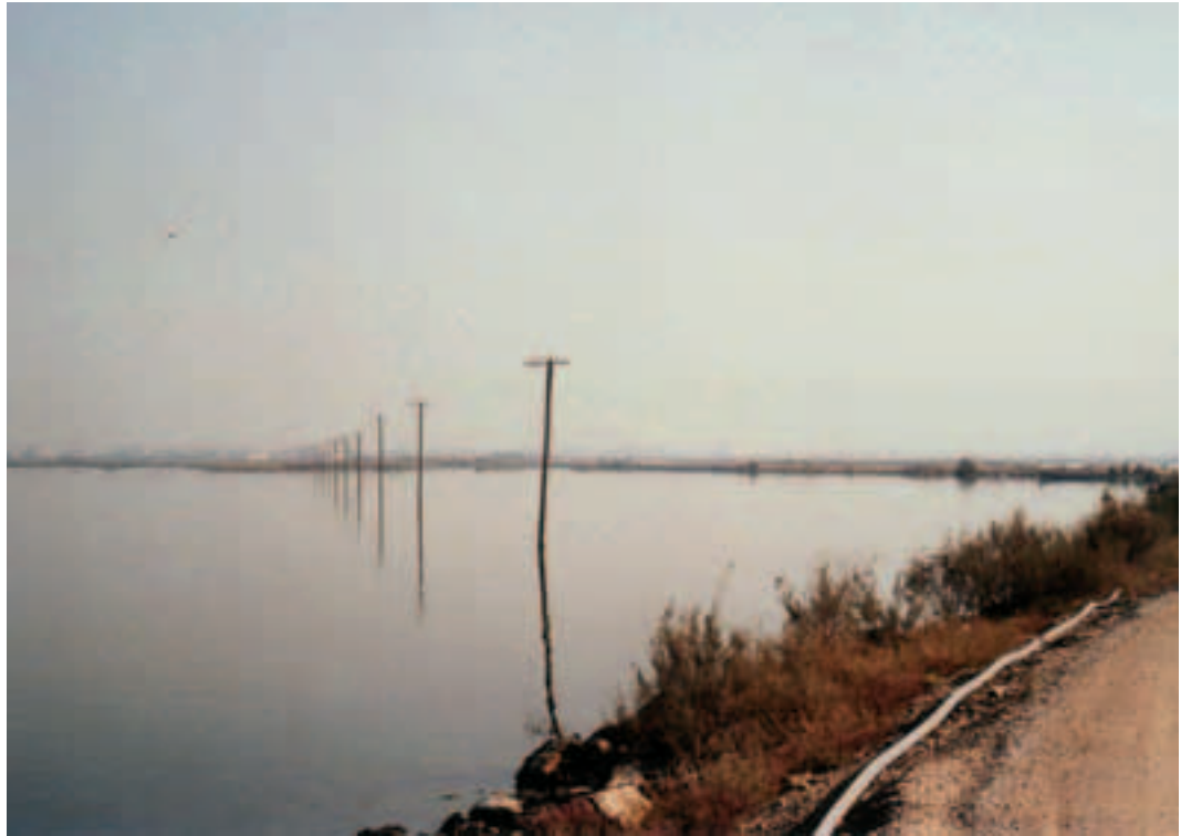
Photo 5.12 - The subsidence is well obvious from the fact that the old road lies beneath the water surface, as it can be seen along the telephone line poles. This happened due to the intensive water groundwater pumping, soil subsidence has occurred and embankments were constructed to prevent seawater intrusion. 8 years ago, one of the dams broke and the sea flooded a large part of the area.
