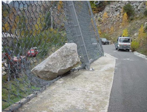
Rock block 2.3 m 3 from the rockfall event of August 17, 2003, trapped by the protection fence of the Forat Negre basin
