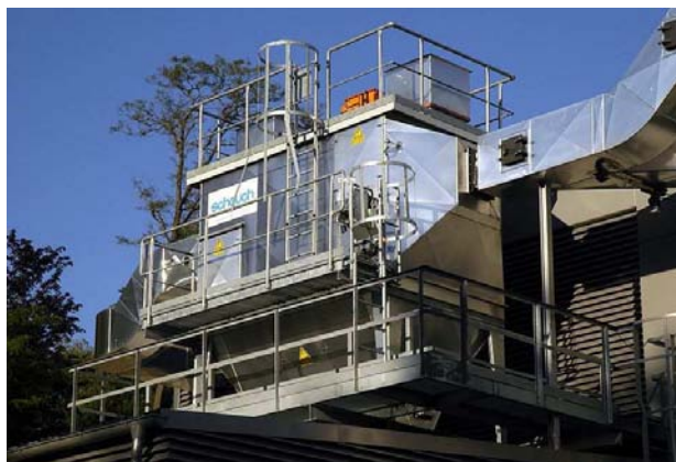
Electrostatic precipitator of a biomass heating system with a heat power of 2 MW (fonte wikipedia)
