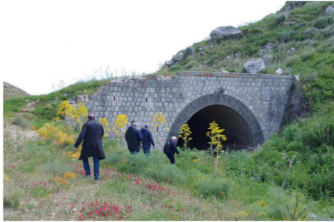
Fig. 17. Entrance upstream of the helicoidal tunnel. The entrance is partially occluded but accessible.
