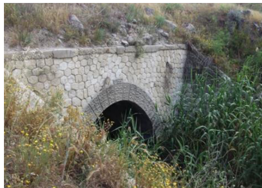
Fig. 16. Downstream entrance to the helicoidal tunnel. It is flooded due to an earthen barrage to store water from a source inside the tunnel.
