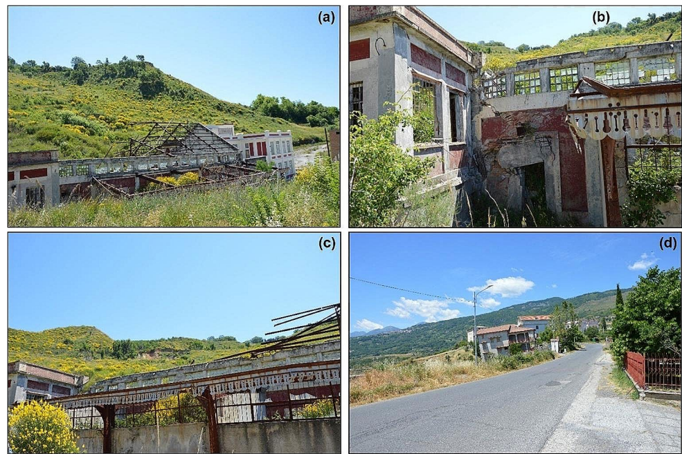
Fig. 1 (a) Panoramic view of the main building of the mine, (b, c) some details of the degradation and (d) a tilted house on top of San Leonardo Hill
