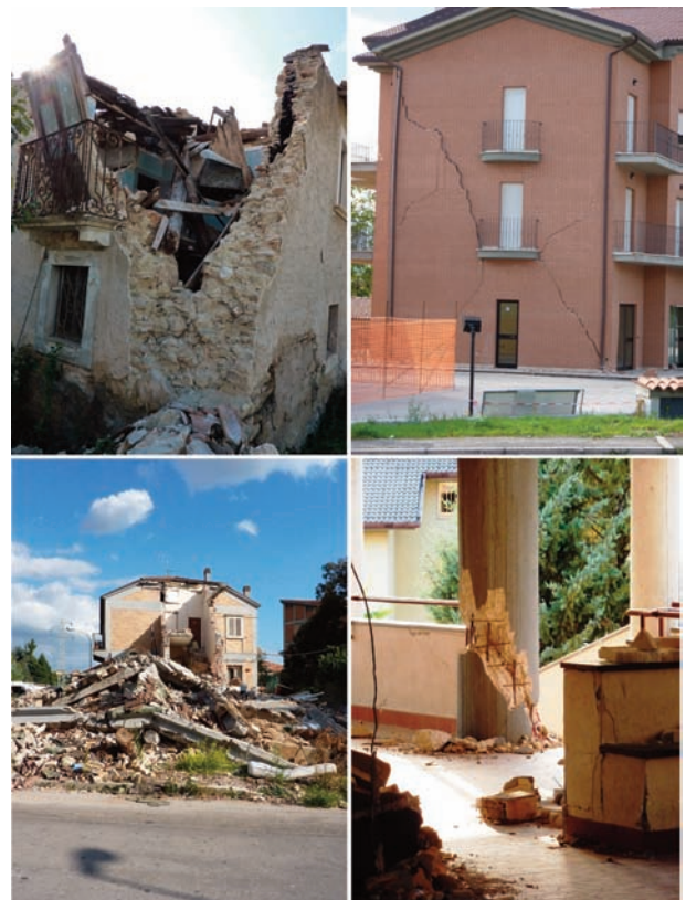
Fig. 1 - 6 April 2009 earthquake damage in private and public buildings of different kinds in L'Aquila, Abruzzi, reflecting the social vulnerability due to poor acceptance of living in a very seismic area.
